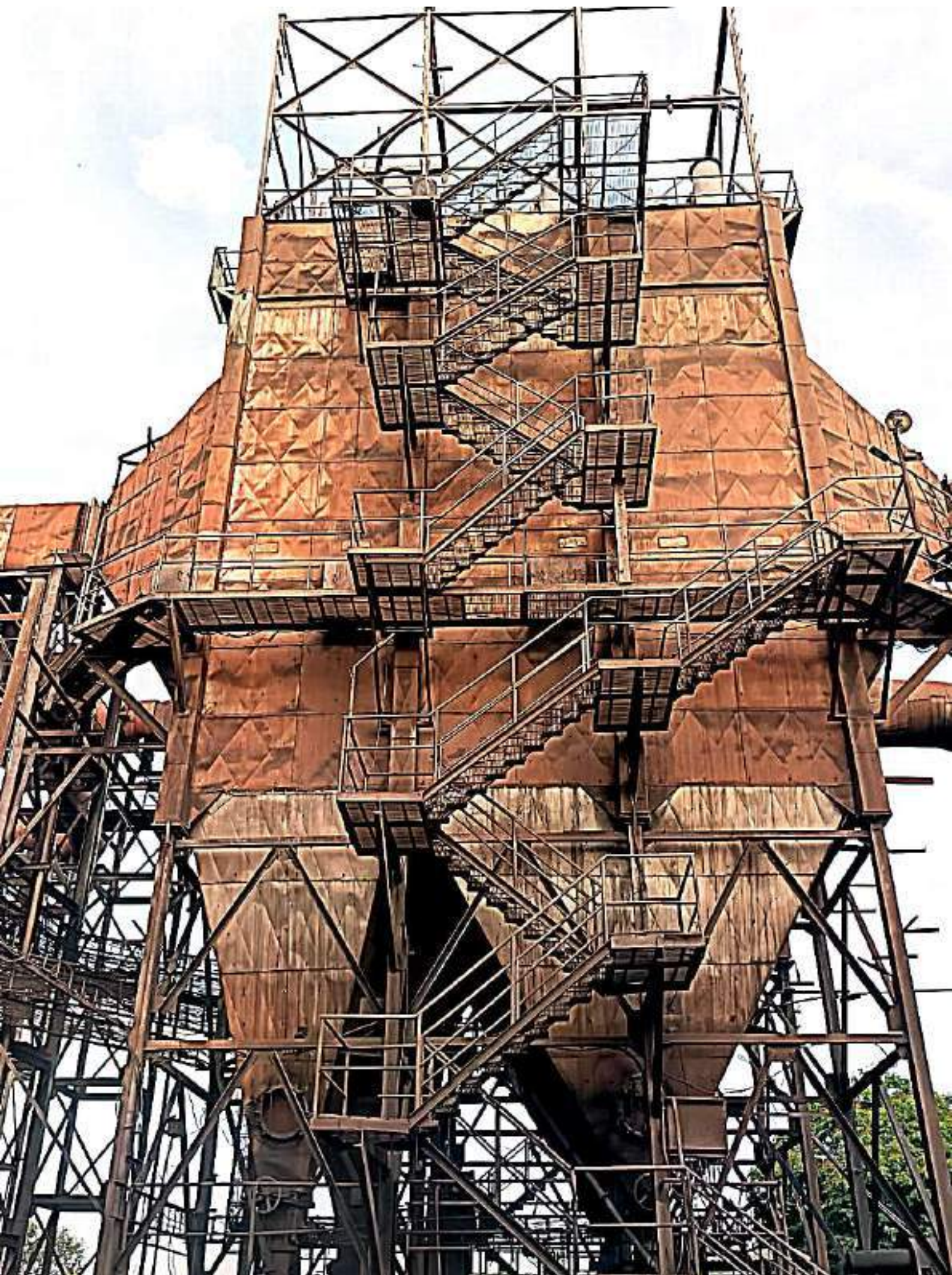
(a) ESP 2 Nos. with common stack
